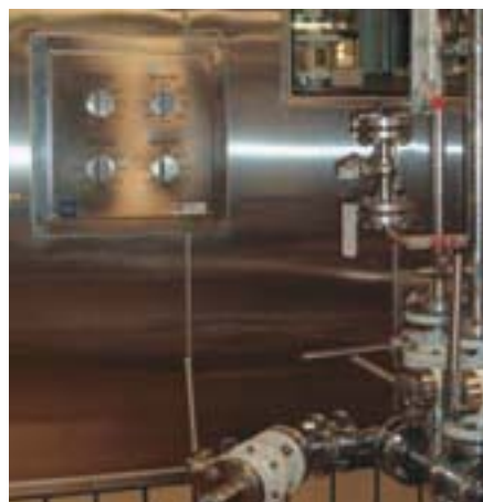
Figure 2: Operator Station on reactor
