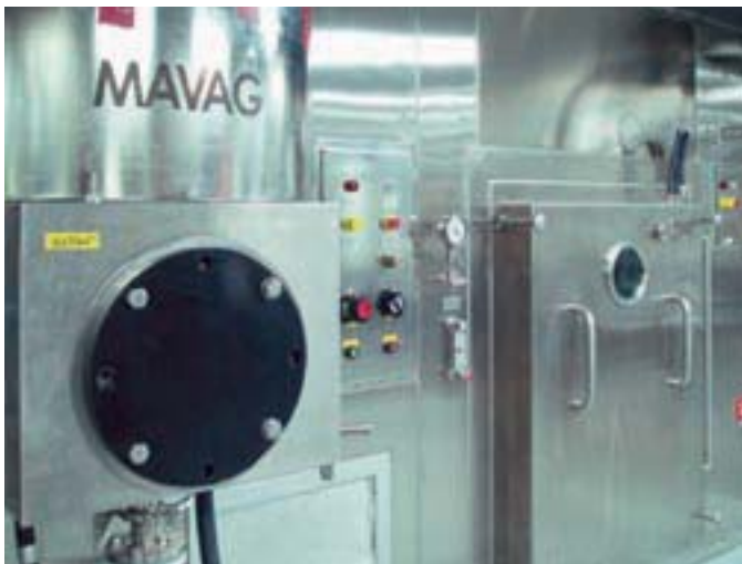
Figure 5: Discharge point on the centrifuge with explosion protected control board
