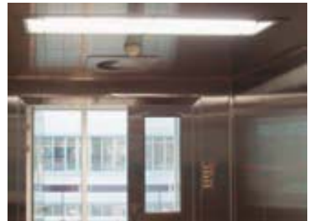
Figure 4: Access lock with explosion protected stainless steel built-in ceiling light fitting
